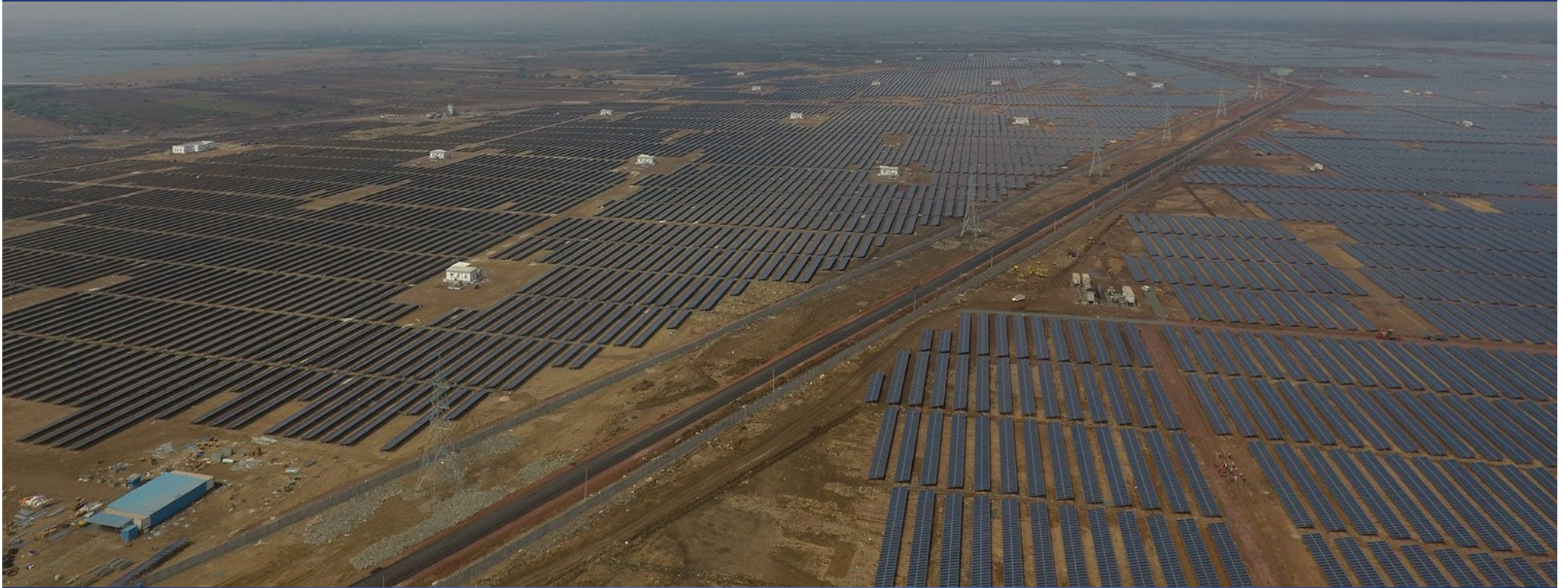
Kurnool Ultra Mega Solar Park, India – 1000 MW, 2017
